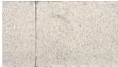
6 Concrete edging strip (600mm wide nom.) in stacked bond pattern in front of entrances
